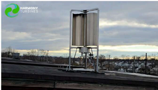
ALPHA unit on Headquarters rooftop
